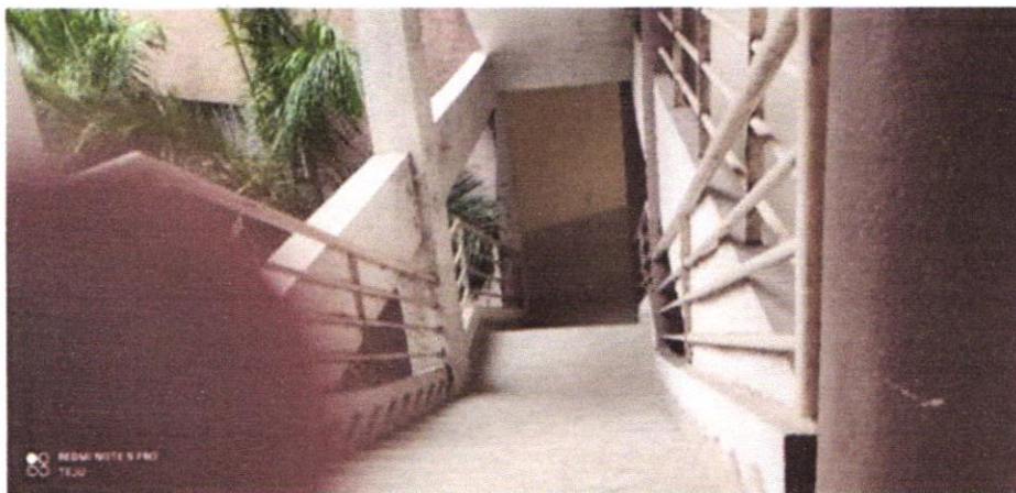
Broad daylight in staircases
